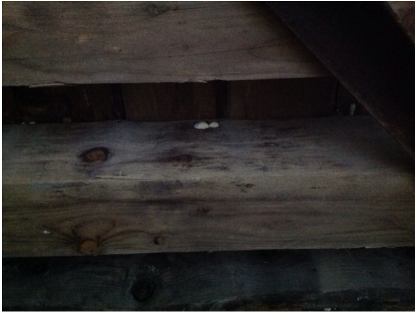
ties starting to show signs of decay
