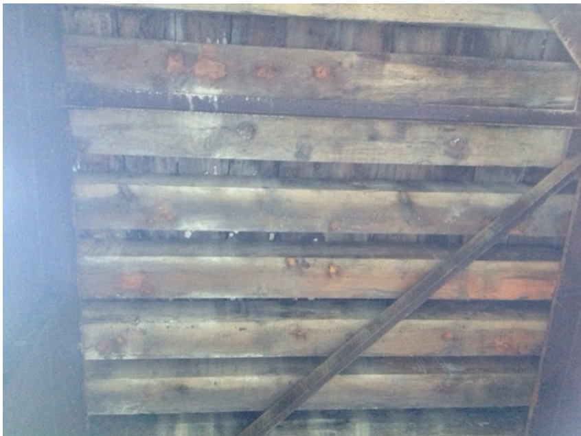
sub deck starting to signs of decay
